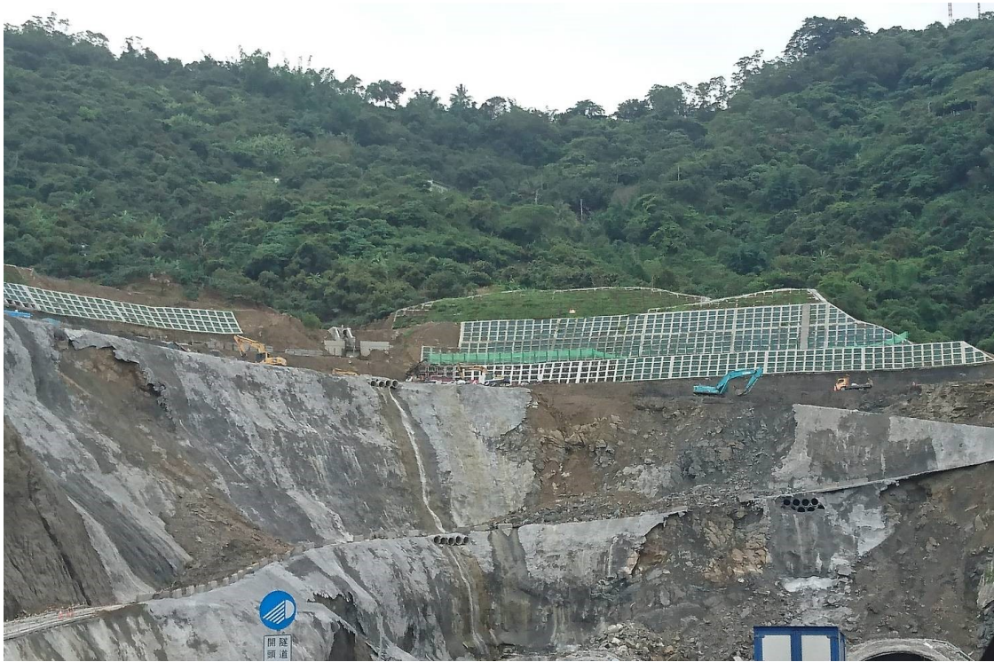
Figure 7. Instability of the slope during the excavation process of the north entrance of the Zhongliao Tunnel into the graben.
