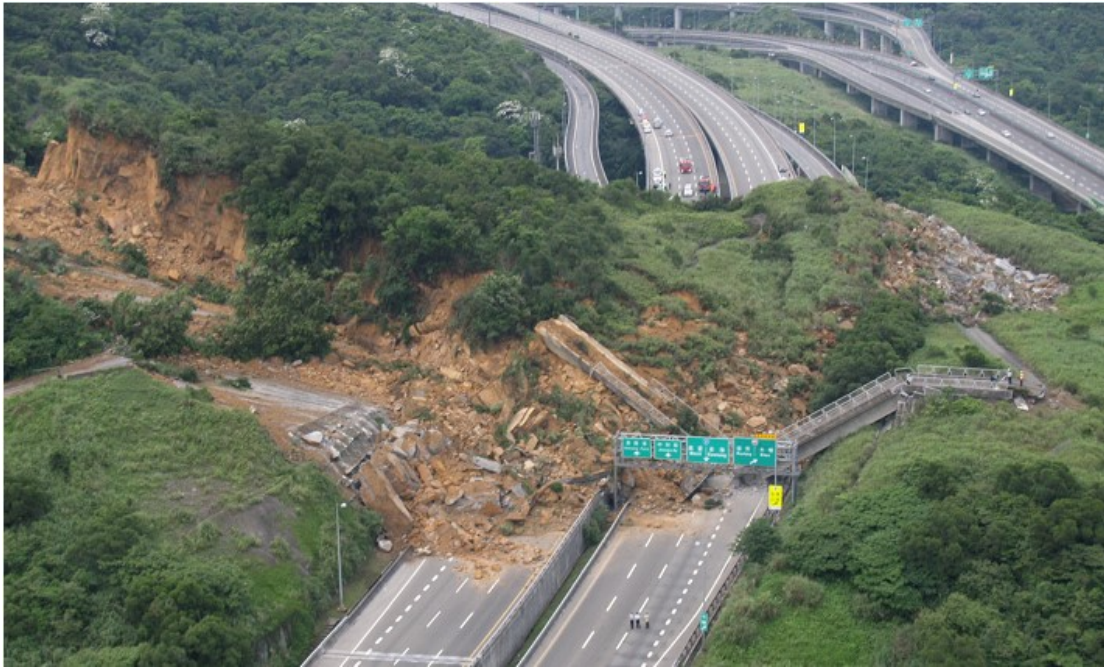
Figure 1. Sliding failure of the anchor retaining wall slope on Formosa Highway No. 3 at 3.1K (Taiwan Geotechnical Society, 2011).
